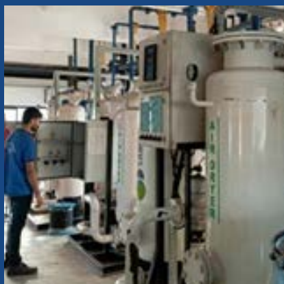
Desiccant air dryer
